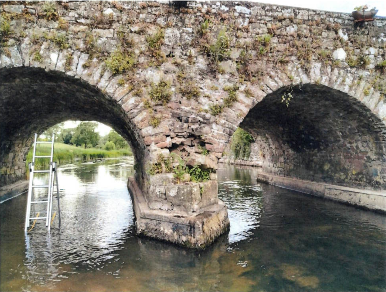
Figure 3. Damaged cutwaters on the upstream side.
