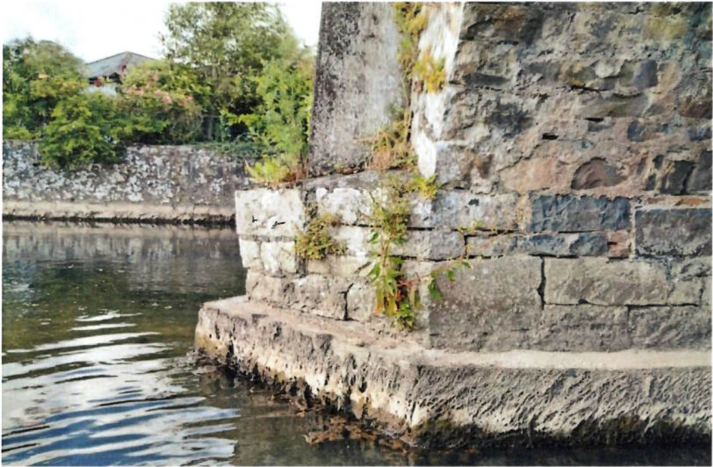
Figure 4. Damaged cutwater on the downstream side.
