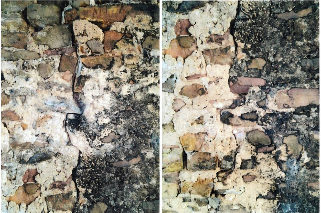
Figure 2. Longitudinal cracks in the arch barrels.
